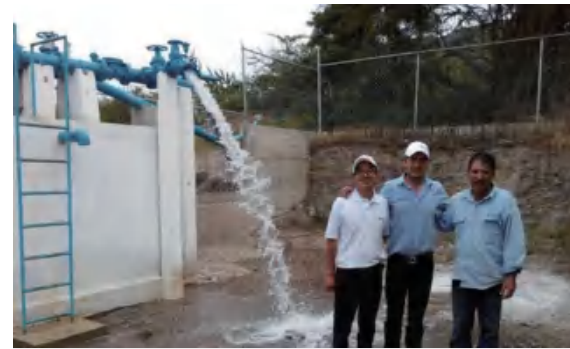
Solution System: 18.5kw System (JNP18K5H) Application: Irrigation Location: Guerrero, Mexico
