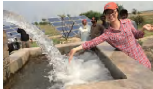
System: 37kw solar pump system Application: Agriculture Irrigation Location: Multan, Pakistan Head: 75m
