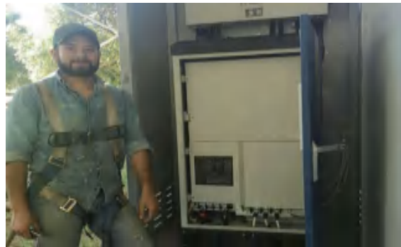
Solution System: 110kw System Application: Irrigation Location: Guerrero, Mexico
