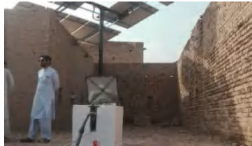
System: 3kw System for NGO Application: Agriculture Irrigation Location: Pakistan
