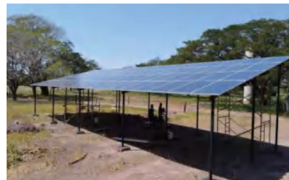
System Solution: 22kw system Application: Agriculture Irrigation Location: Colombia
