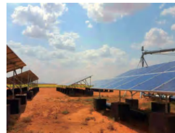
Solution System: 55kw Solar Pump System Application: Daily Water Supply & Irrigation Location: Sudan
