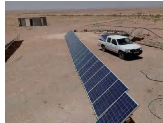
Solution System: 2.2kw System (JNP2K2L) Application: Livestock Drinking Water location: Algeria
