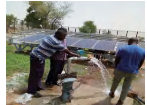
System Solution: 13 set 1.1-7.5kw System (UNDP project) Application: Drinking & Irrigation Location: Sudan
