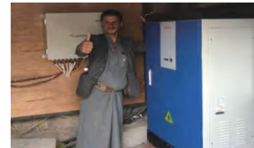
System Solution: 75kw system NICEF-Operate Solar Pumping System for Tlwmos Well – Sadah. Location: Yemen
